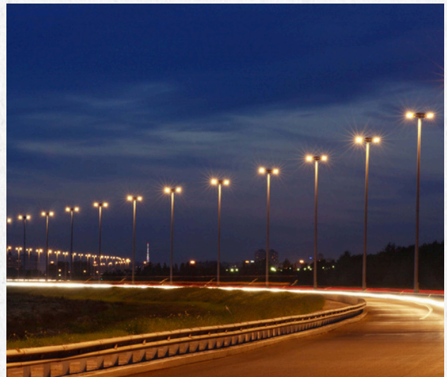
ROAD & HIGHWAY LIGHTS
